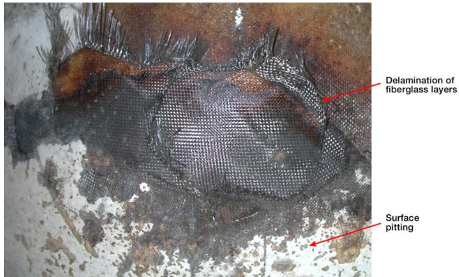
Figure 3.2-22. Delamination and pitting damage.
